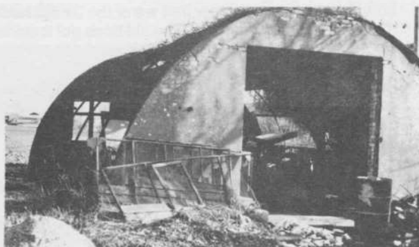
Nissen hut being cleaned up and a new roof will be installed.
